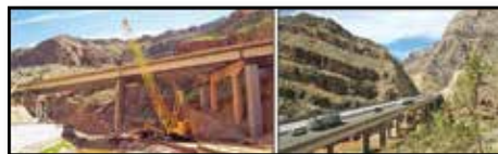
Figure 11. One of the seven bridges constructed in the gorge. Most have undergone retrofitting and upgrades since they were originally completed in the early 1970s. ADOT photos.
